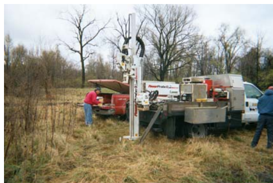
Soil and Groundwater Sampling With a Push-Probe Drill Rig at the Subject Property
